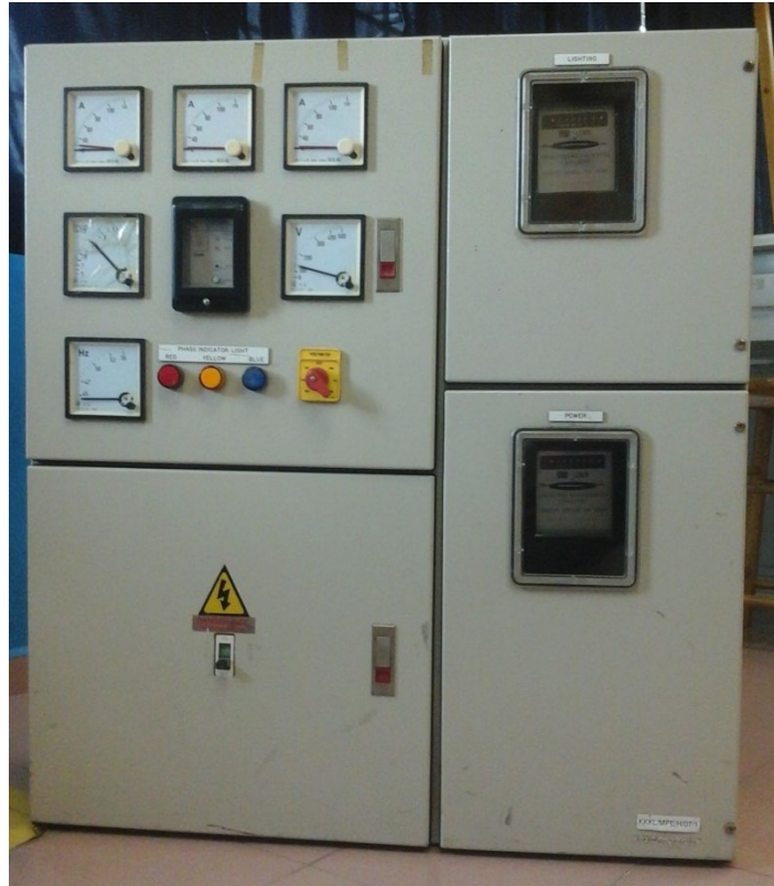
Rajah 5: Sub Switchboard
